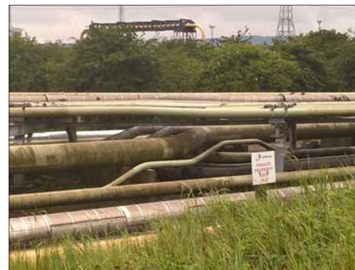
Sembcorp link lines
