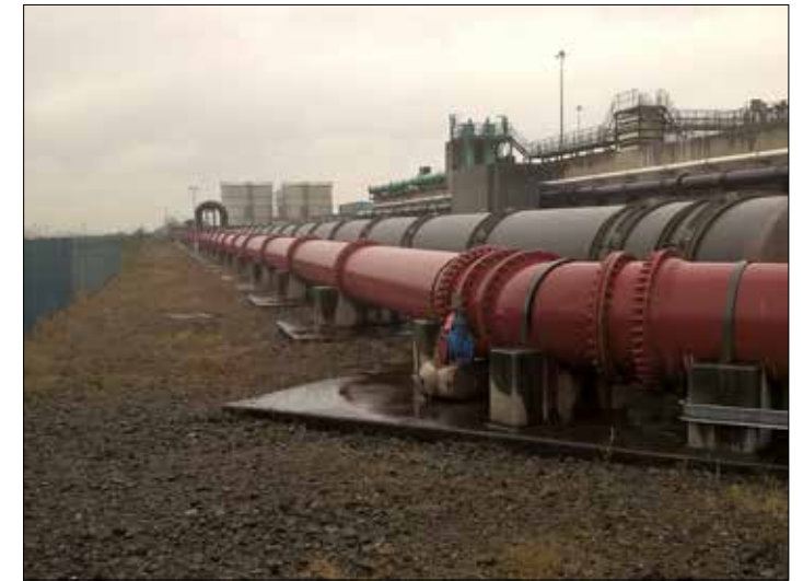
WWTW Sewage Transfer Mains
