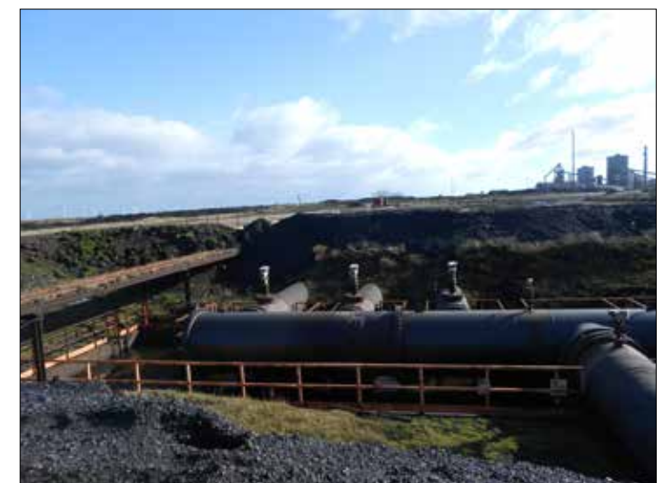
RBT - Estuary water mains - Valve chamber
