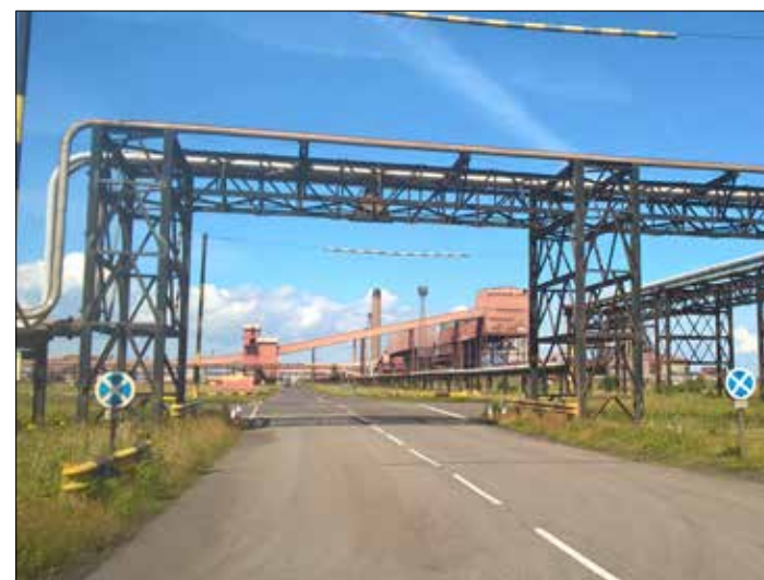
Redcar - COGM and Heavy Fuel Oil line crossing
