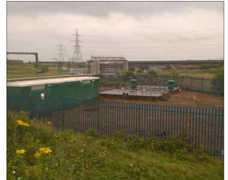
Eston Pumping Station Sewage Transfer Mains
